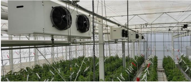
Hi-Tech (Air condition)
