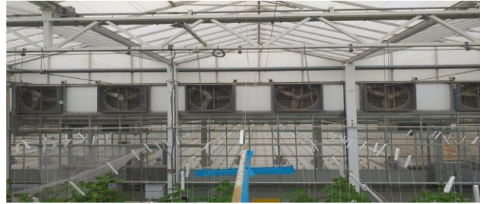
Med-Tech (Pad and Fan)
